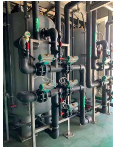
Mixed Bed Resin Tower
