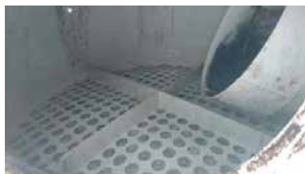
Cleaning Air Pollution Equipment Tower
