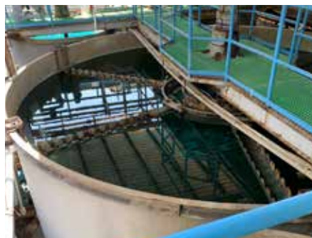
Wastewater Treatment System
