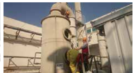
Regular Maintenance of Air Pollution Equipment
