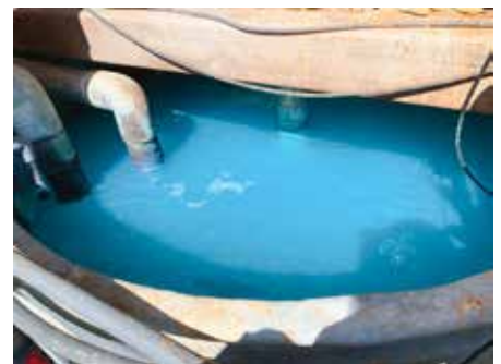
Wastewater Treatment System
