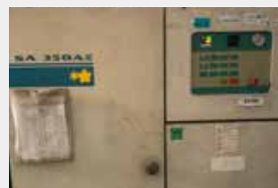
Decrease the air supply pressure of the air compressor system to reduce the power consumption
