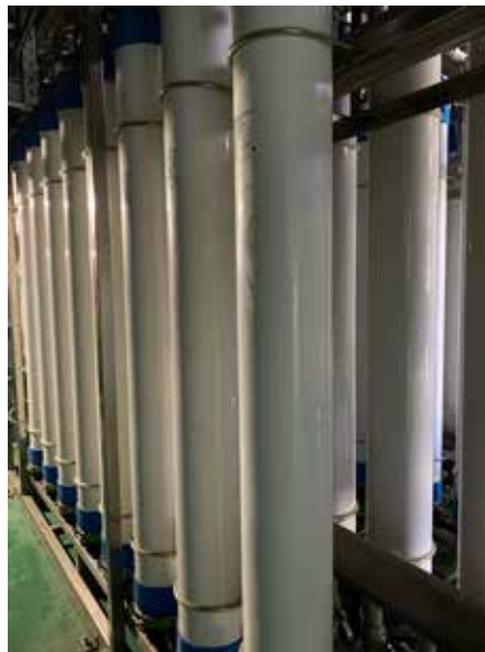
RO Membrane Tube of Recycled Water
