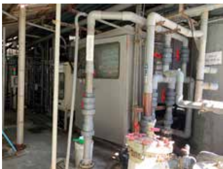
Wastewater Treatment System
