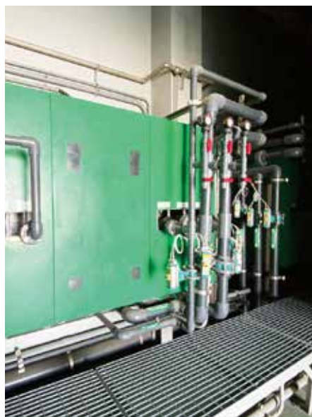
Reclaimed water treatment facility electrodiolysis reversal (EDR) unit
