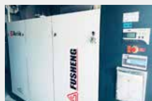
Replacement of two traditional compressors with a frequency conversion one
