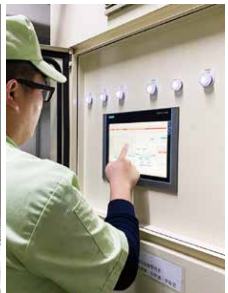
Reclaimed water treatment facility automated control system
