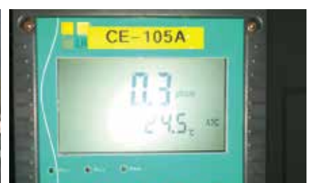
Purified water conductivity monitoring
