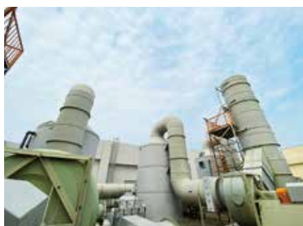
Air pollution prevention system
