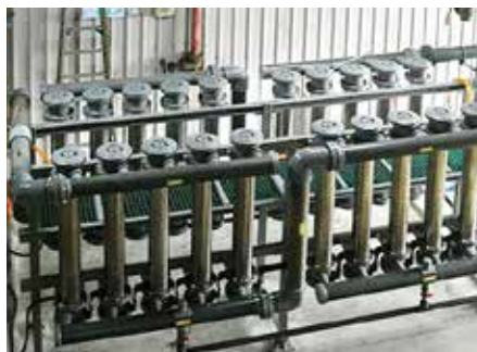
Electrolytic copper recovery system
