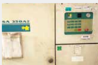
Adjust air pressure supplied by air compressor to reduce electricity consumption
