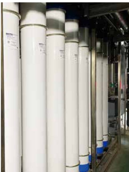
Reclaimed water treatment facility ultrafiltration (UF) unit
