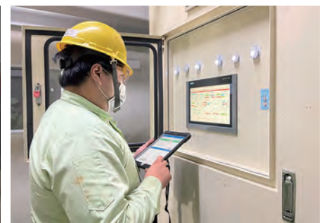
Automated controls for the reclaimed water system
