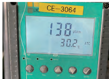
Reclaimed water quality monitoring
