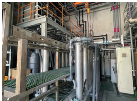
Electrolytic copper recovery system
