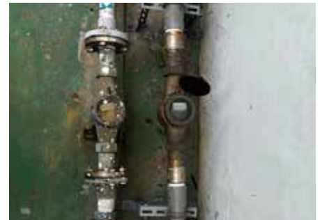
ROR Cooling Towers/Wet Scrubbers Switch and Meter
