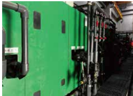
EDR Waste Water Recovery System
